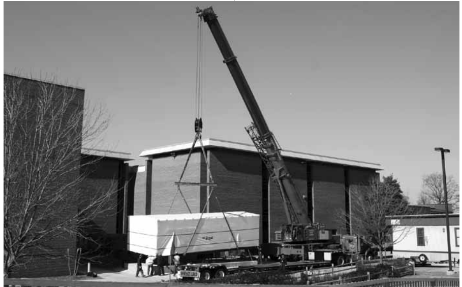
Wiley|Wilson designed a 13.8kV campus power distribution system that used an automated intelligent piece of switchgear, the installation of which is shown here at a community college in Maryland.
