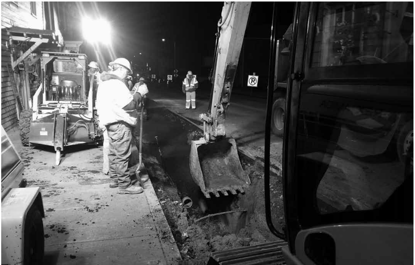
Town crews worked at night to keep disruption of traffic to a minimum.
