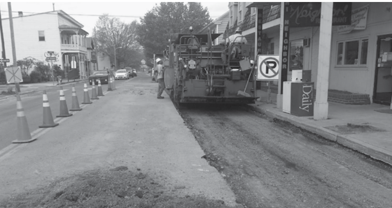
Town crews were able to complete the labor-intensive project within its 11-week schedule.
